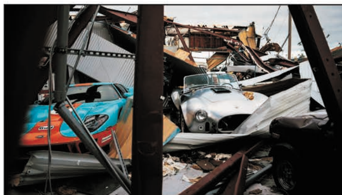
A metal frame building after hurricane Michael... not a good thing for your classic cars.
